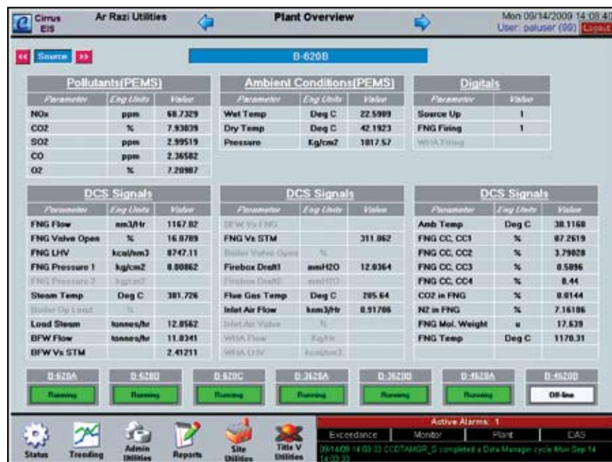
FIGURE 5. This typical DAS reporting screen shows the status of all input parameters for one of the seven boilers. The green boxes at the bottom of the screen show that six of the seven boilers are running and one is shut down
